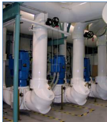
District Cooling Project, Phoenix, U.S.A.
